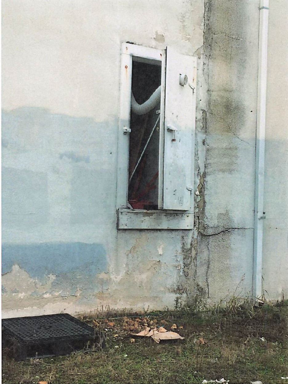
Side exit improper egress.
